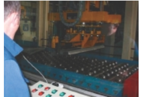
Parkegate designed and supplied this scrap handling system.
